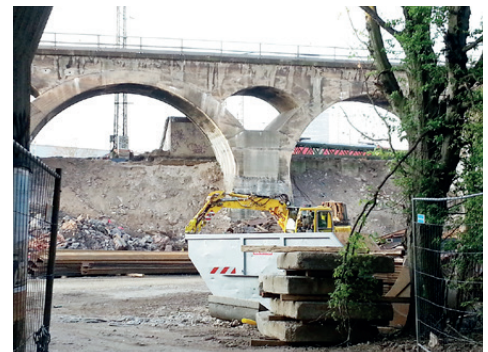
Existing railway bridge in Cologne in need of renovation. Copyright: Obermeyer.
